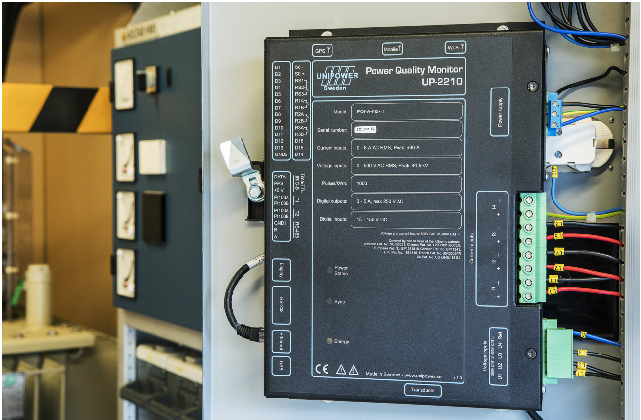
UP-2210 connected to 3CT and 3PT.
