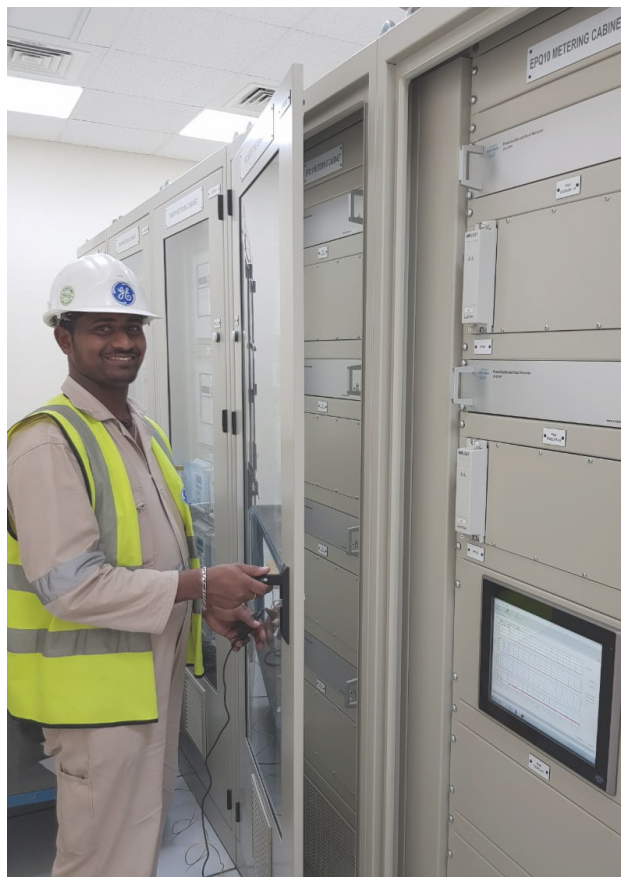
Substation display connected to UP-2210R.
